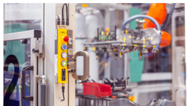
Safety chaining of all safety doors
